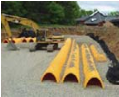
Example of Infiltration Practices Underground storage and infiltration, Bradshaw Celebration of Life Center — Stillwater, MN
