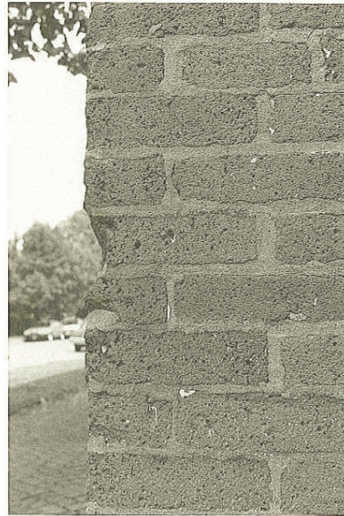
[Photo 9] Brick that has been sand blasted. Note the loss of corner definition, the porous surface, and the weathering that has occurred as a result of sandblasting.
