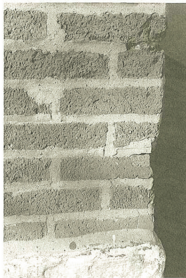
[Photo 10] Sandblasted brick. In addition to the typical damage shown in Photo 9, this example has mortar joints that are both incorrectly tooled and irregular in size and profile.
