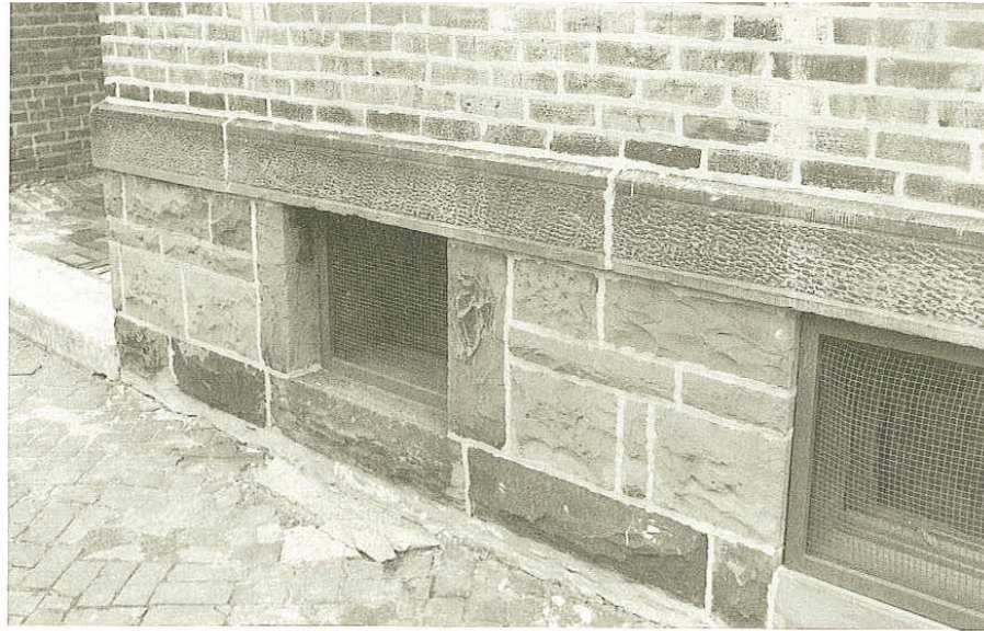
[Photo 2] A rock-faced limestone foundation with a tooled and edged stone water table.
