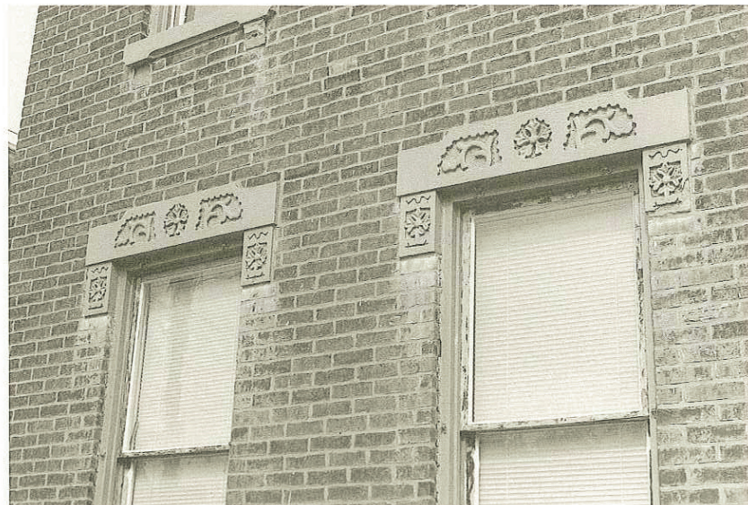
[Photo 33] Although many have been painted over the years, cut-stone lintels such as these were designed to remain unpainted.
