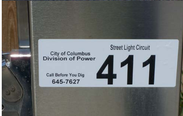
Overhead Utility Cable Line Markers and Pole Tags
