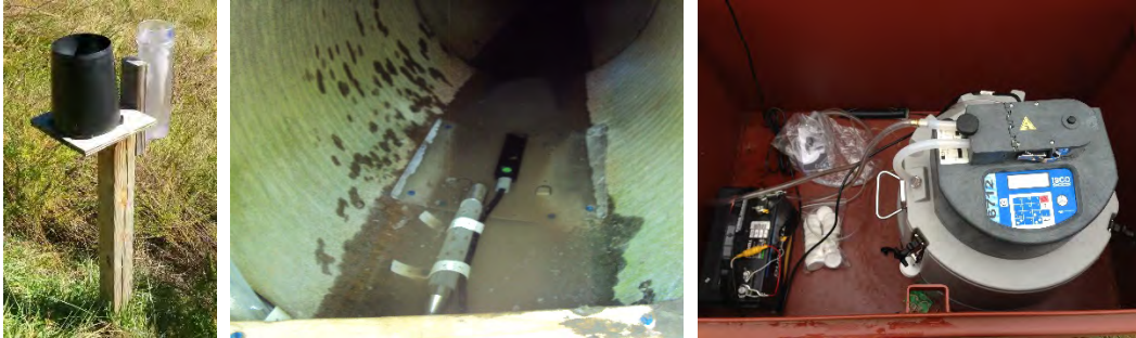
Figure 2. Rain gage setup (left), sample intake (clear plastic) and area velocity meter (black) in the Cooke-Glenmont outfall (center), and automated sampler at Beechwold (right).
