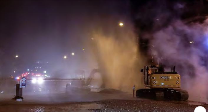
DISPATCH.COM Water-main break spews five-story geyser in downtown Akron AKRON — City of Akron officials say no one was injured this weekend wh...
