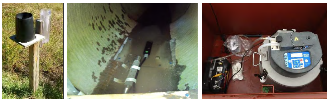
Figure 6. Rain gage setup (left), sample intake (clear plastic) and area velocity meter (black) in the Cooke-Glenmont outfall (center), and automated sampler at Beechwold (right).
