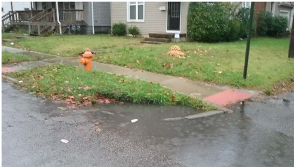
Figure 2. Drainage problem at southwest corner of Eureka Avenue and Grace Street Intersection
