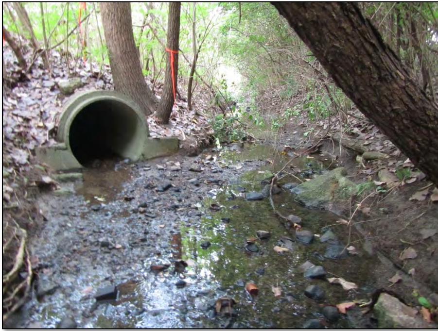
Photo 5: Incoming storm water pipe connected to Wetlands A & B in interchange islands.
