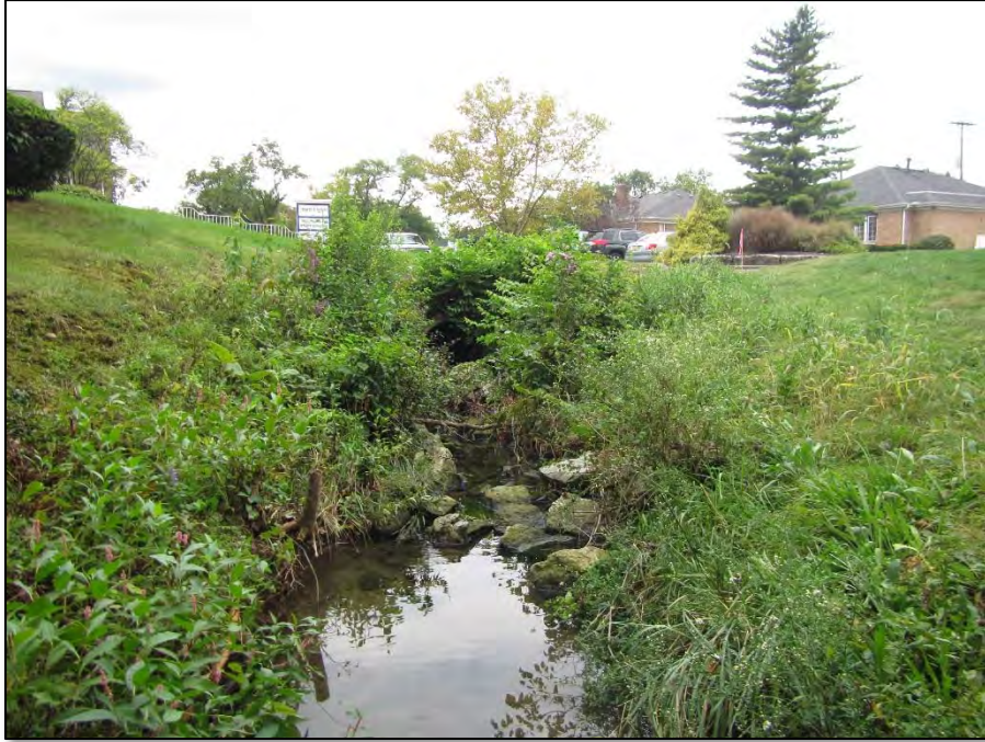
Photo 1: Looking upstream at head of unnamed tributary emerging from culvert on adjacent property.
