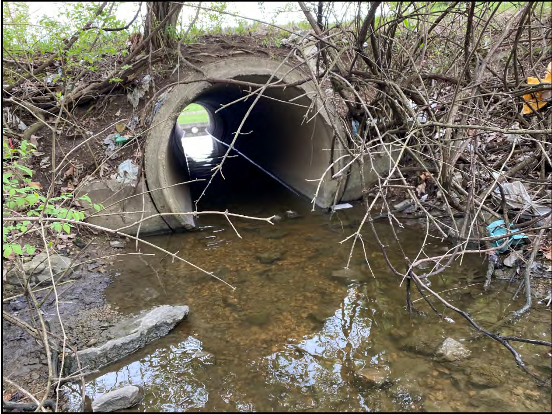
Photo 29 – Westerly view at the origination of Stream 9. This culvert pipe discharges surface water from a west adjoining storm water management pond.
