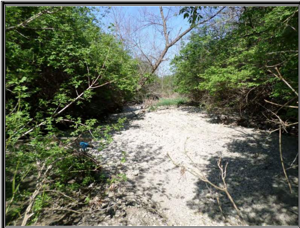
Photo 26 (4/20/16): Northeasterly view along the drainage channel as it traverses the southern portion of the property.
