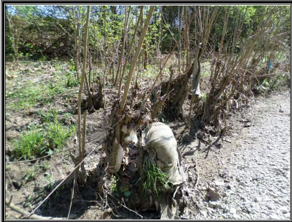
Photo 29 (4/20/16): View of drift deposits visible along the edge of the channel on the south central portion of the property. The drift deposits indicate the channel does accept heavy, fast flow of short duration during significant rain events.
