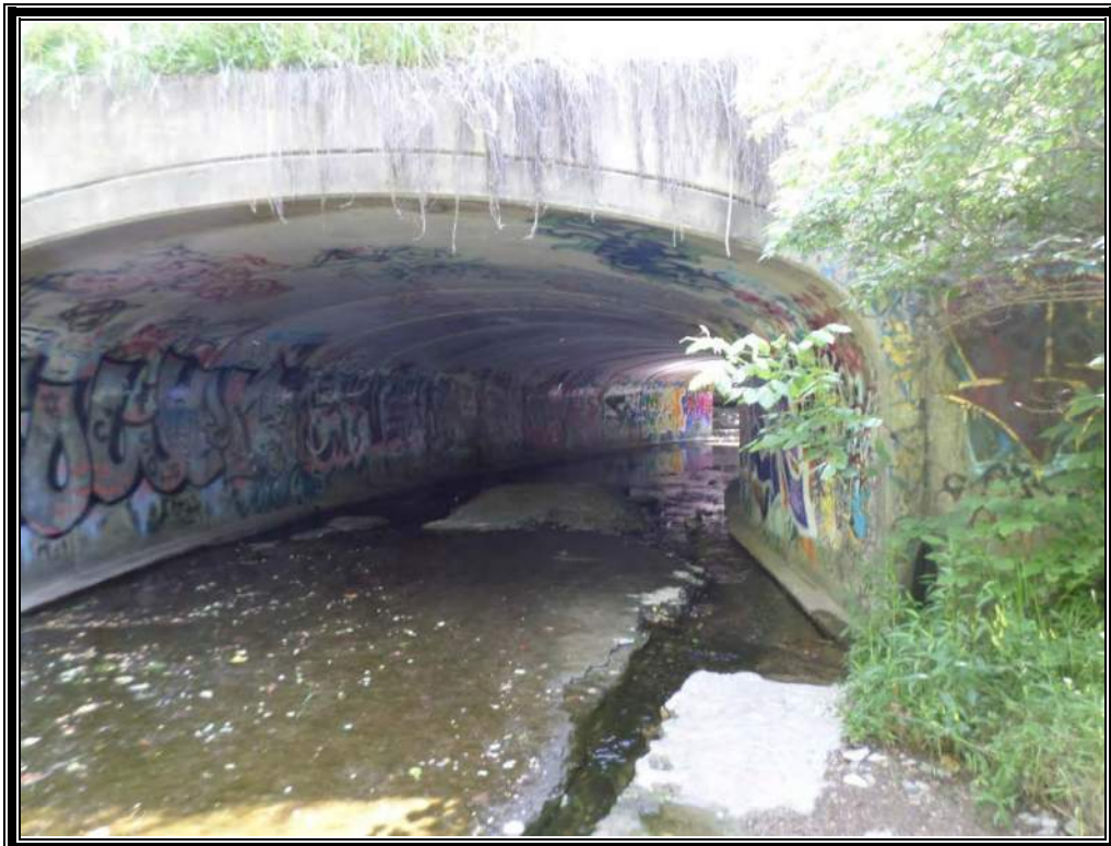
Photo 4 (6/14/16): Easterly view along Roberts Millikin Ditch and the culvert beneath Dublin Road. This photo is from off-site, west of Dublin Road.
