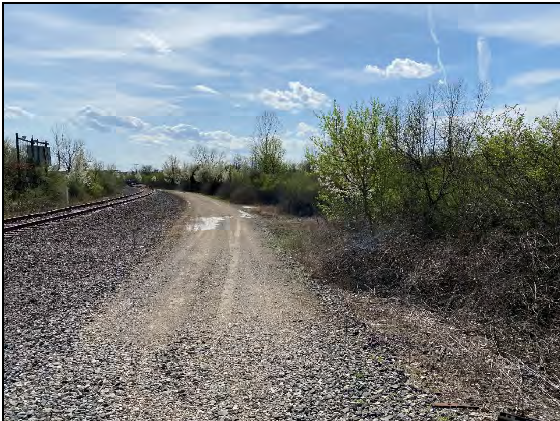
Photo 2 – Typical view of former rail lines and adjacent brushy areas on the North Section of the evaluation area.
