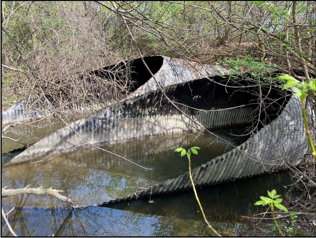
Photo 17 – Northeasterly view of two existing culvert pipes directing surface water from Stream 1 (Roberts Millikin Ditch) beneath elevated railroad lines.
